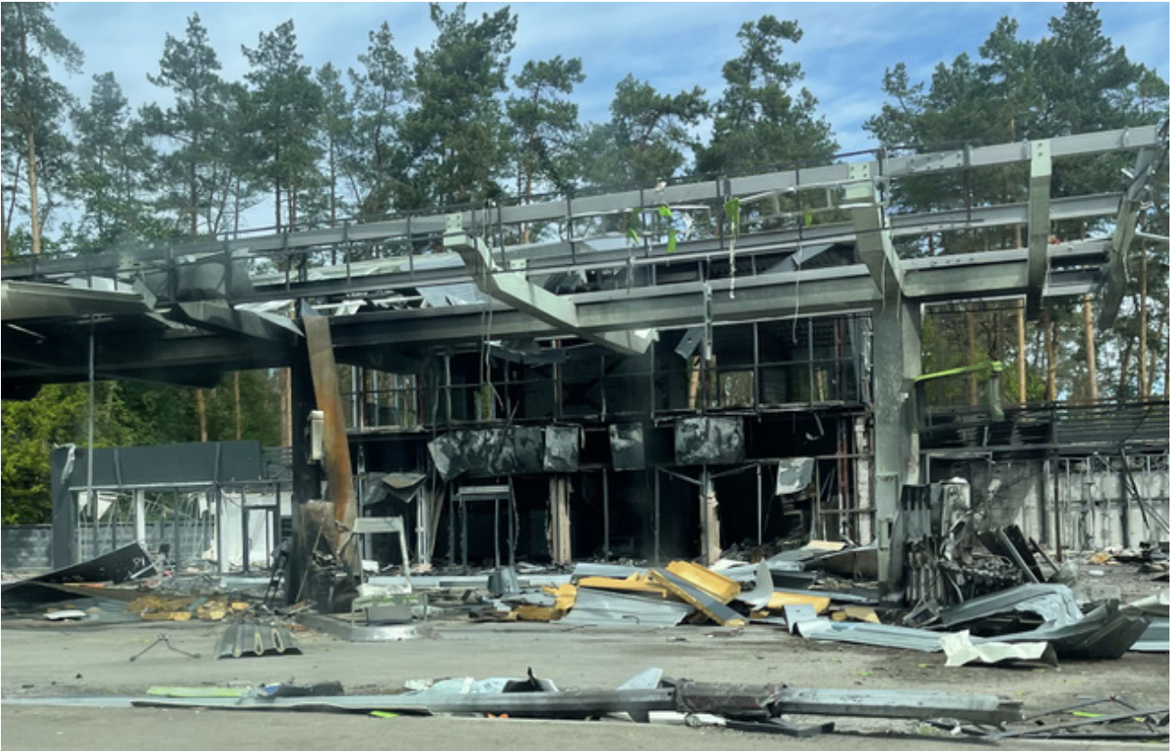
One of the many petrol stations that were bombed, cutting off fuel supplies for residents. Image source: Lam Bao Yan
