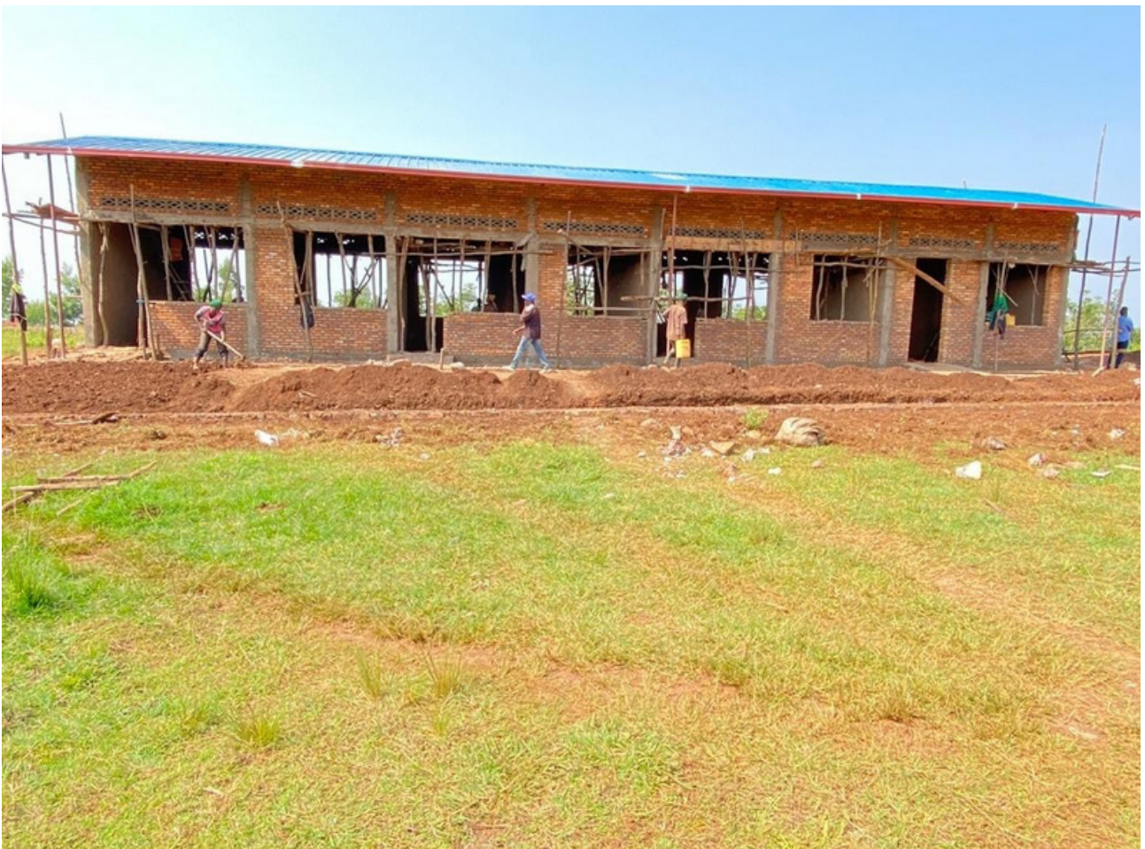
A building project in Rwanda. PHOTO: Rudy Taslim and Lam Bao Yan
